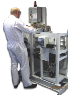
PET Cyclotron Facility Stack Monitoring - Lab Impex Systems
